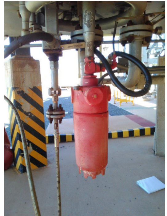
Existing Fireeye 45UV5 Series flame scanners at gas plant
