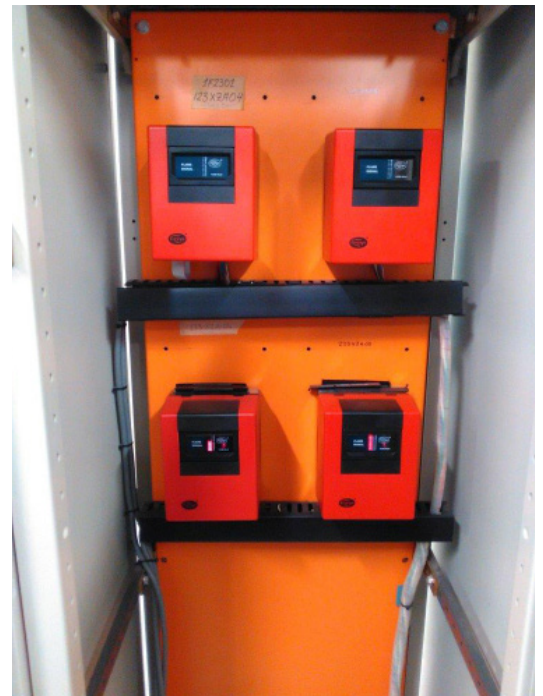
Existing Fireeye Flame-Monitors at gas plant
